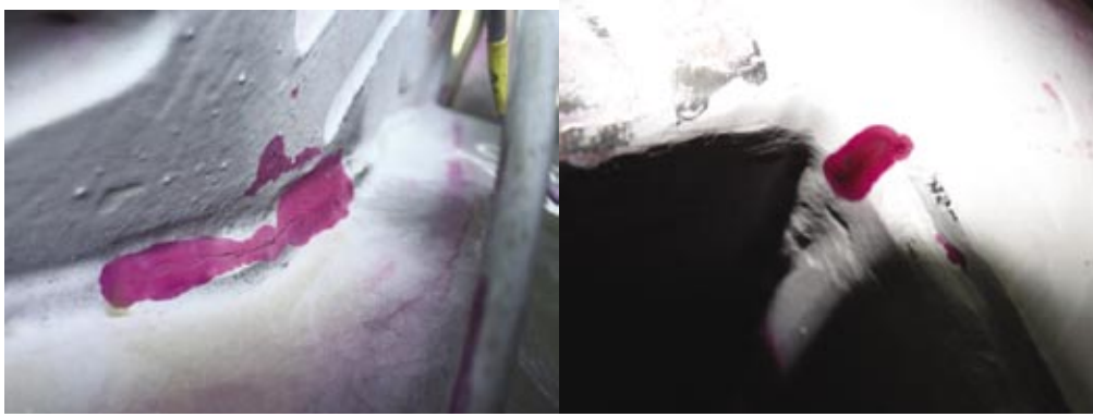
Fig. 6. Examples of joint penetrant testing results – welding imperfections in the form of cracks
