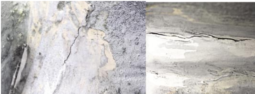
Fig. 7. Examples of joint MT results – welding imperfections in the form of cracks
